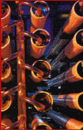
Reverse osmosis water filtration equipment, Marco Island, Florida.
