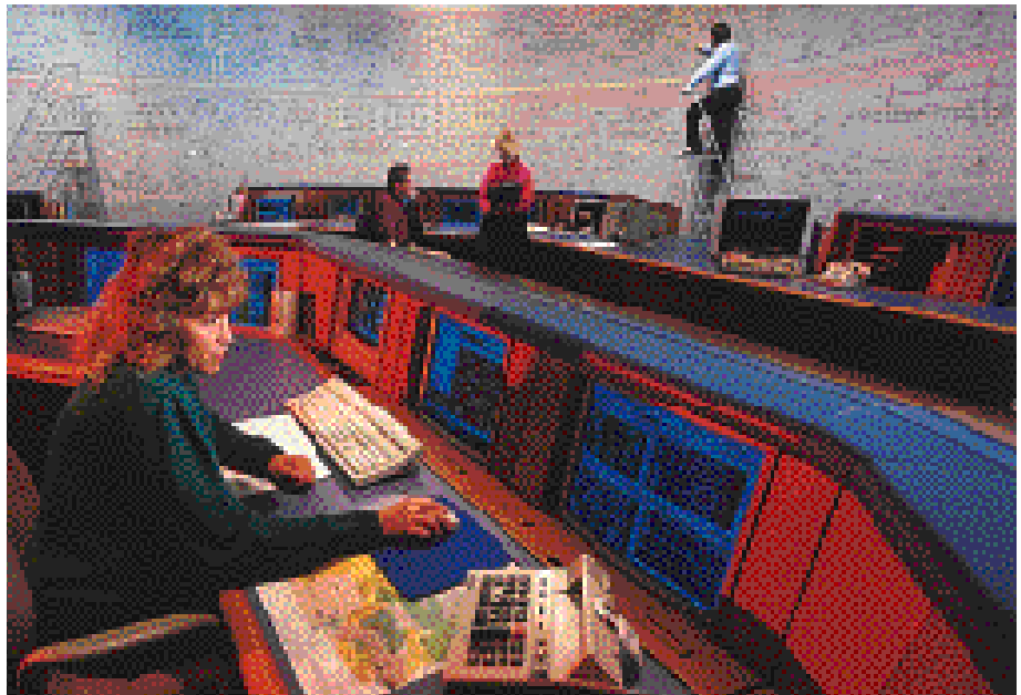
System Operator Christine Laskowski uses a state-of-the-art control system to monitor MP Electric's power grid from the Rowe Energy Control Center in Duluth.
